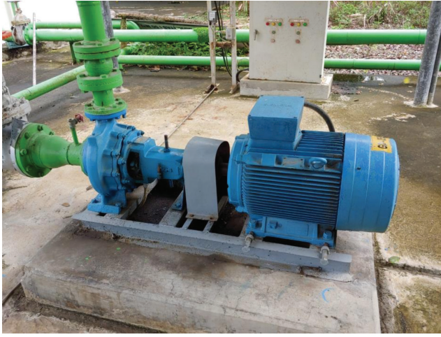
Gambar 1. Pompa Potable Water
