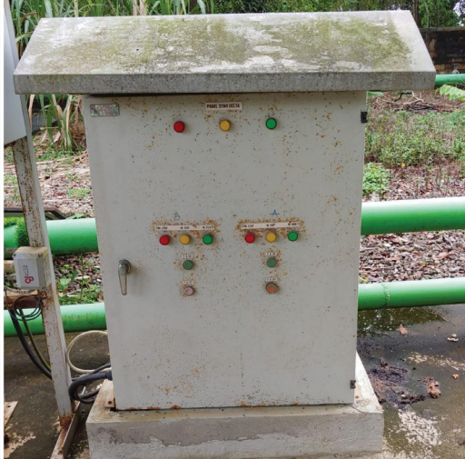
Gambar 2. Panel Variable Speed Drive
